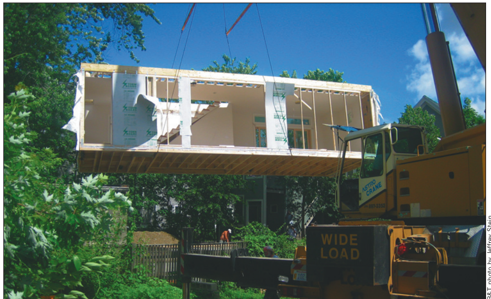
A crane lifts one-quarter of Christine Cuttita and Bob Gillig's modular house – including framing, sheathing, roof, doors, windows, inside plaster, plumbing and cabinets – onto its site on Harris Street in Somerville. The husband-and-wife team is the creative pair behind Somerville's Cuttita and Gillig Architecture.
